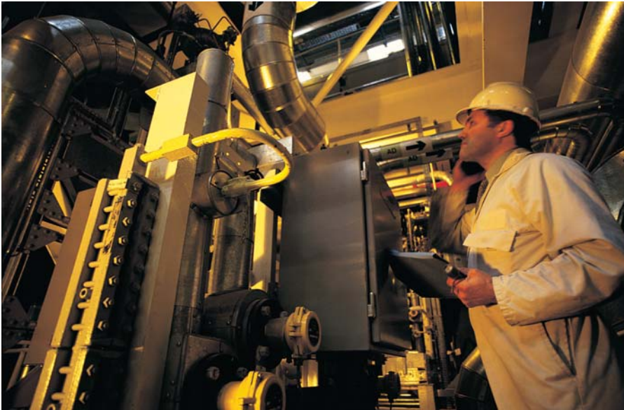
HMI terminals make maintenance easier by giving access to all information from one point.
